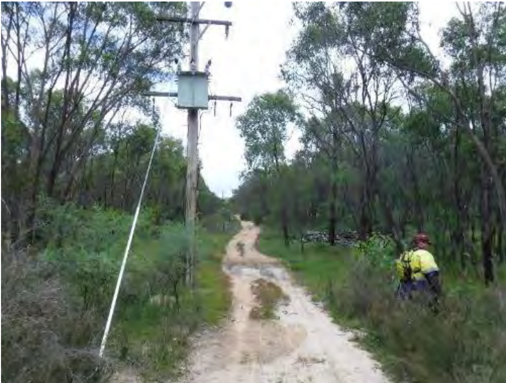
Photo 3.6 Existing transmission line
