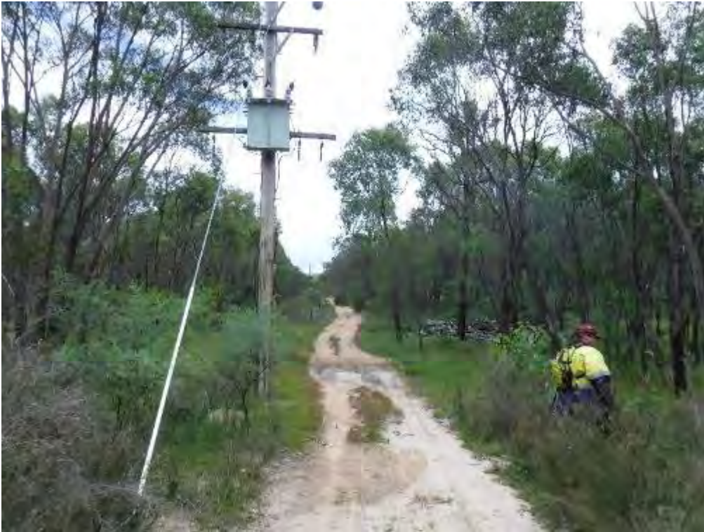
Photo 3.6 Existing transmission line
