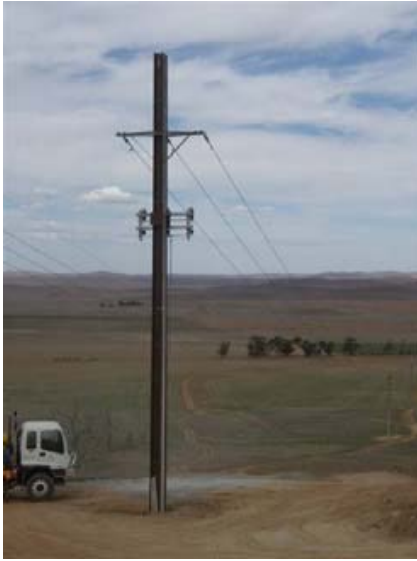
Figure 2.4 33 kV overhead feeder lines
