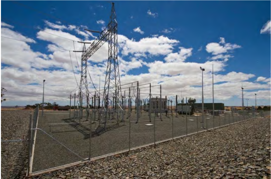
Figure 3 Example of a substation with the gantry in the foreground
