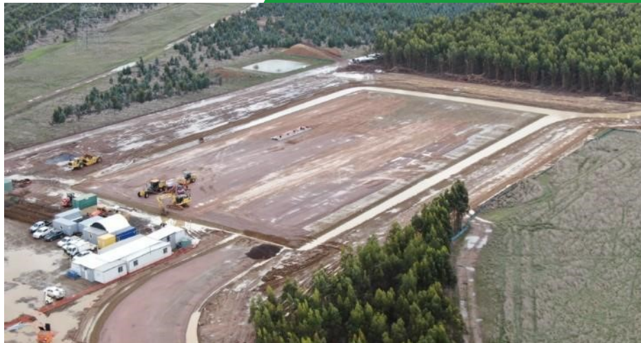
Blue Gums Substation pad and site compound
