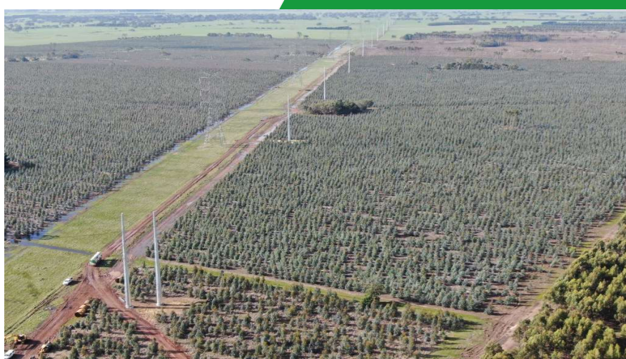
Poles nearest to the Blue Gums Substation
