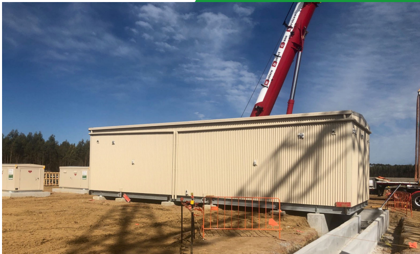
Control room delivered to Blue Gums Substation
