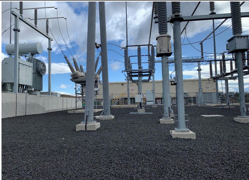
Photo 9: Project Collector Substation.
